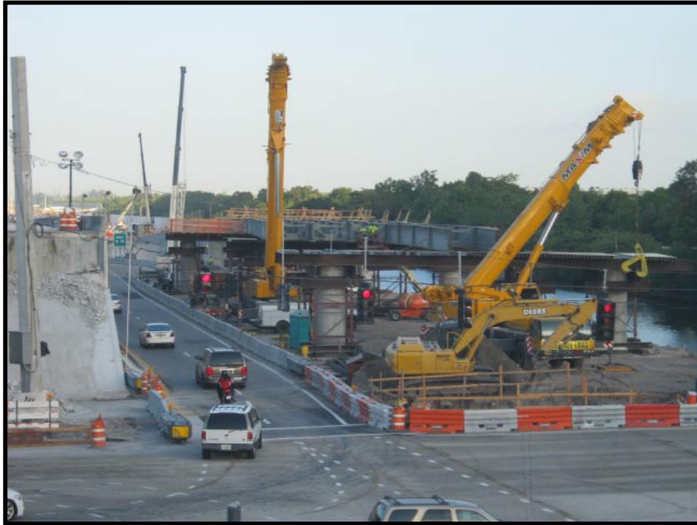
Ongoing ramp construction at the northwest corner of Pine Island Road and S.R. 84
