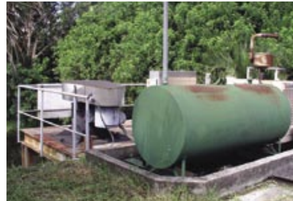
Dated and deteriorating pump station to be replaced
