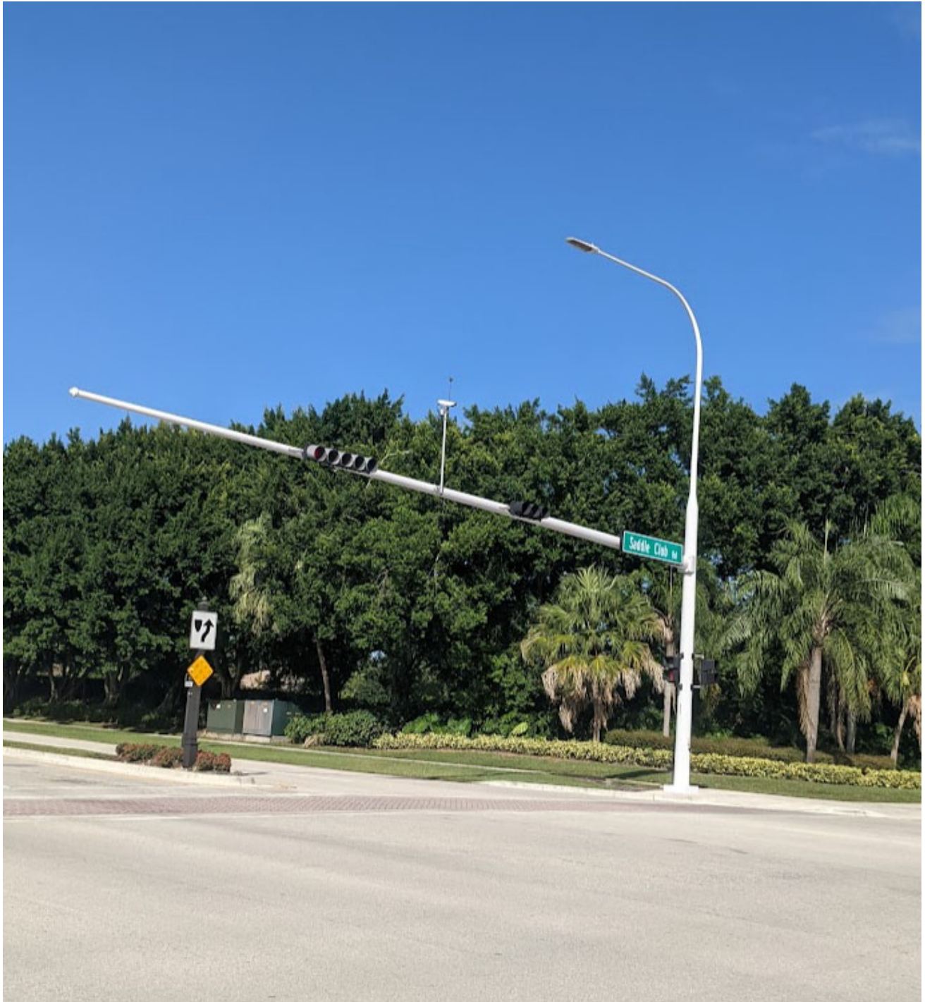
Mast Arm Assembly with Streetlight Arm
